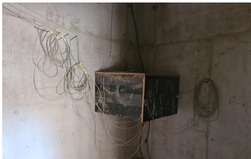
Figure 52. Box containing data acquisition equipment
