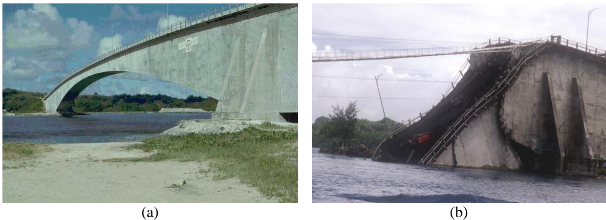
Figure 20. (a) Koror-Babeldaob bridge after construction; (b) Koror-Babeldaob bridge after collapse
